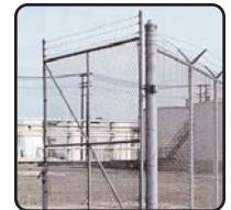
Perimeter Vibration Sensors, Motion Sensors
